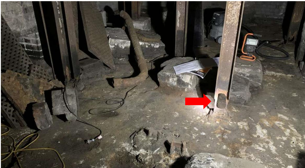
Figure 5. Steel columns support the cast iron grates at the floor above, and all are suffering extreme corrosion particularly at their base, meaning that the grates are non-trafficable and at risk of collapse.
