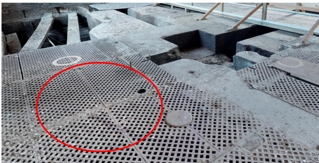
Figure 2. The cast iron floor grates present an asbestos hazard, with their porous surface containing remnant fibres despite previous cleaning in the room. Note also the large cavities present across parts of the floor. The hygienist has described that it would be implausible to fully clean the grates of asbestos in-situ, given the myriad openings and porous surface.
