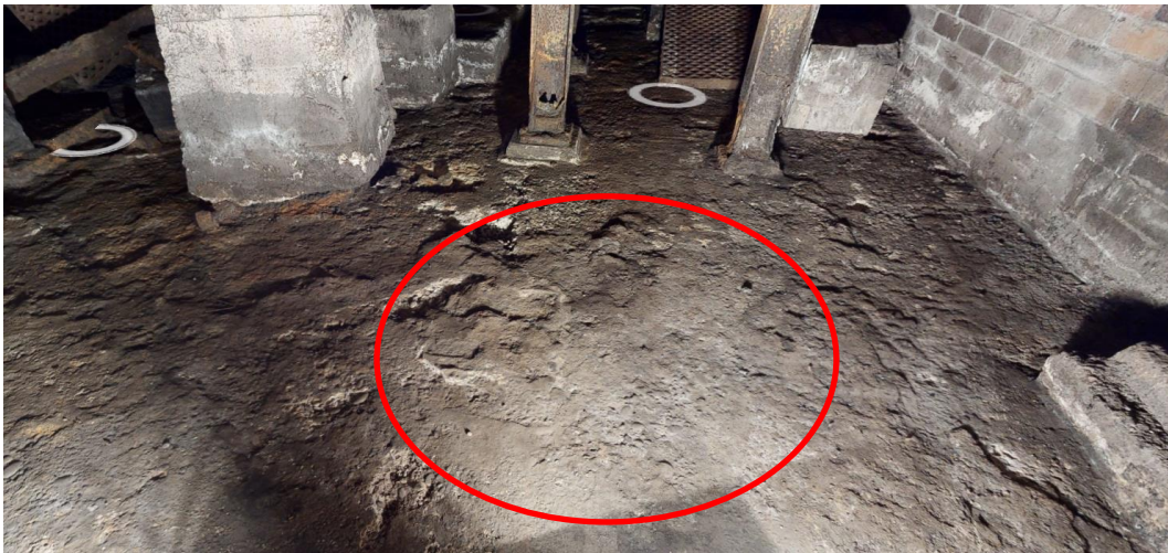
Figure 4. The solidified base surface however presents an asbestos hazard, with detectable asbestos physically embedded within the surface material.
