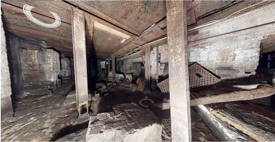
Figure 3. A very deep sub-floor cavity is present below the grates, which has been cleaned of asbestos as best as possible.
